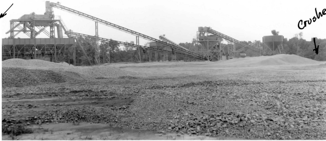
View of the plant assembly from the north west corner of the stockpile area.
