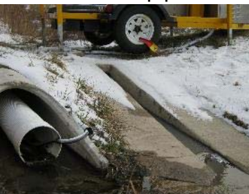
7i. TB19gw 8-in. underdrain pipe
